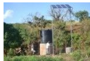
To make the best use of the reservoir, solar powered pumps were installed at our wells.
